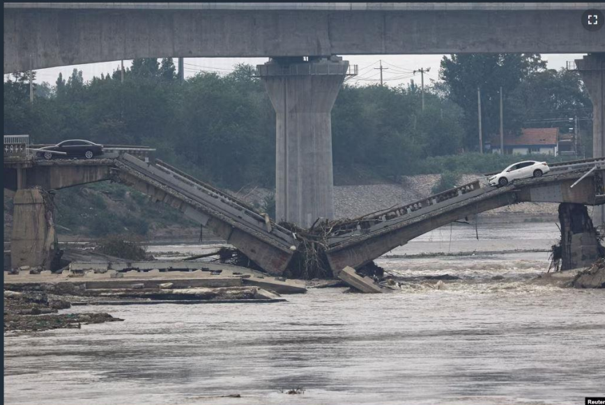
4 A bridge is damaged after remnants of Typhoon Doksuni brought rains and floods in Beijing, China, Aug. 2, 2023.
